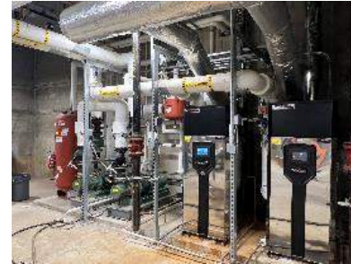
Hot Water Boiler Plant
