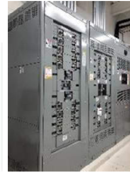
New Service Equipment
