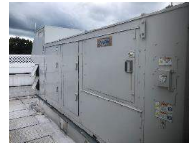
Rooftop Ventilation Unit
