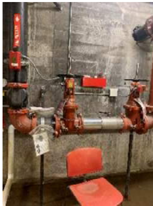
Existing Sprinkler Service Valves
