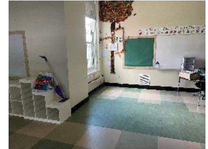
Perimeter FTR Heating
