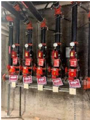
Existing Sprinkler Zone Control Valves
