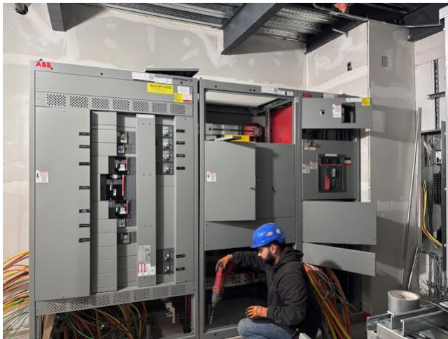
Electrical Switch Gear Installed in the Main Electrical Room
