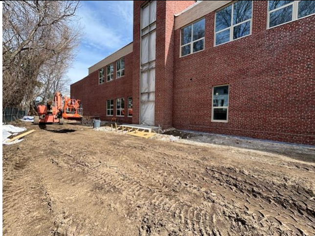
Brick Veneer Completed Along the West Elevation and Curtainwall Framing Installed at Stair 8
