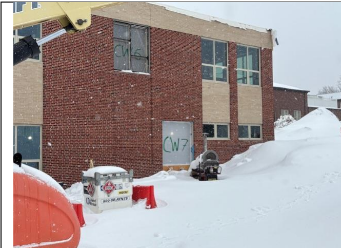
Windows and Curtainwall Installed along the South Elevation of the South Addition
